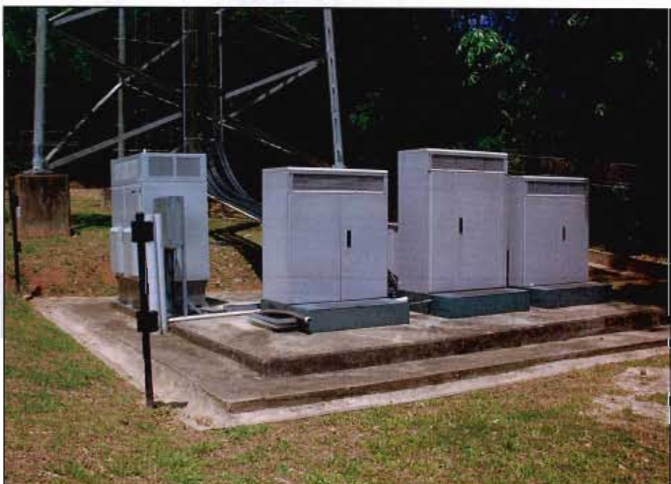
With a fuel cell system that has an integrated fuel reformer and a fuel tank (in the cabinet to the left), when the grid power fails at a wireless telecom site, a small battery string takes over the site's load for a couple of minutes while the fuel reformer starts up and produces hydrogen, and then the fuel cell begins powering the site's load (the three base stations in the other cabinets).
