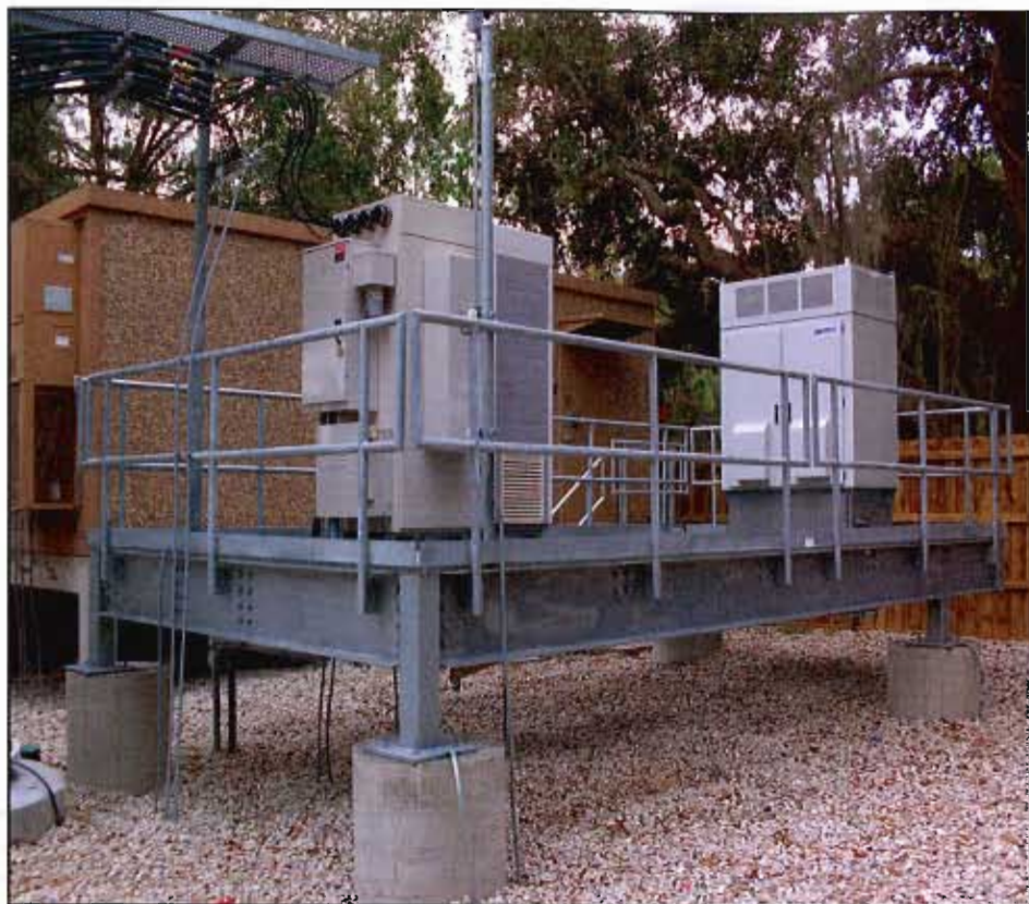
An alternative to the traditional backup electric power for telecom installations has become commercially available: the fuel cell. A fuel cell, housed in the cabinet to the right side of the platform, produces electricity through an electrochemical reaction.
