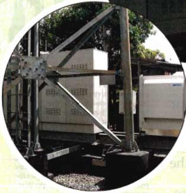
Indonesia base station site with backup power fuel system.
